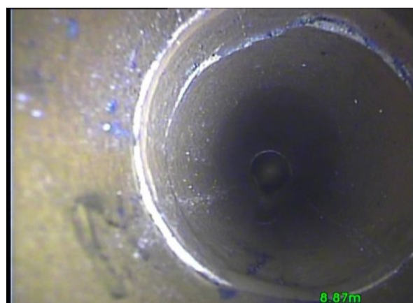
4, 00:00:58, 8.86m Fracture, circumferential from 9 o'clock to 4 o'clock
