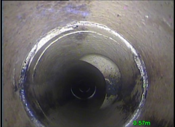
1, 00:00:17, 0.57m Fracture, circumferential from 12 o'clock to 12 o'clock
