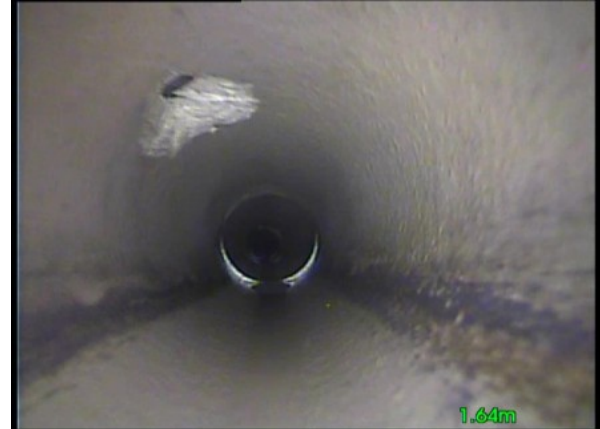
2, 00:00:22, 1.64m Hole in drain or sewer at 11 o'clock
