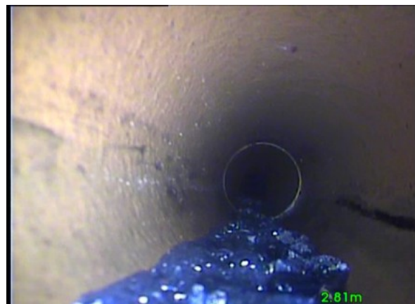
2, 00:00:25, 2.80m Settled deposits, coarse, 5% cross-sectional area loss, start
