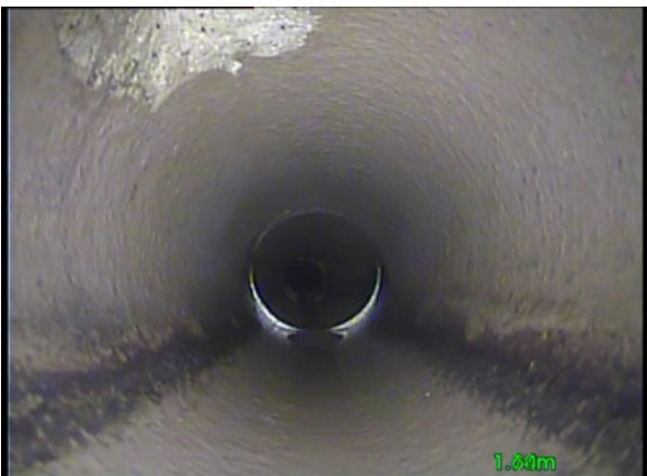
3, 00:00:22, 1.64m Hole in drain or sewer at 11 o'clock
